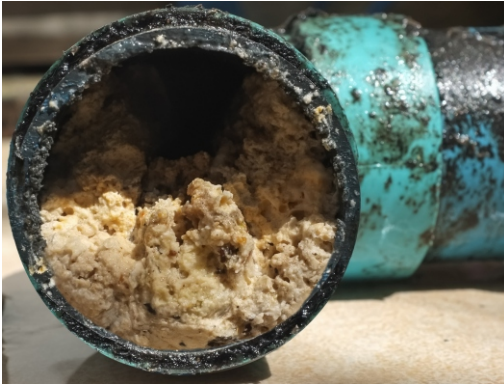
ABOVE: Actual photo of build-up of fats, oils, and grease in a sanitary sewer.
